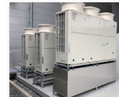
冷凍機置場①
